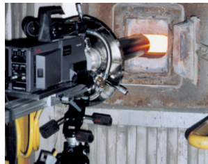
Special high temperature vortex tubes keep a boroscope lens cool while inserted into a 1200°F (650°C) boiler porthole.
